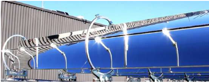
RACK10: rooftop collector
