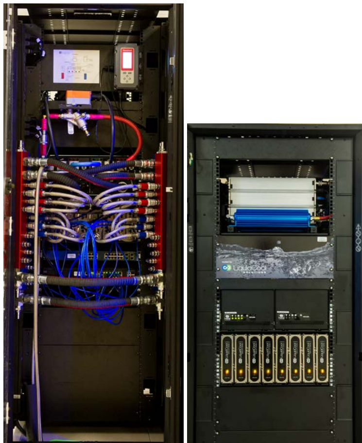
Figure 26. Left: Eight-server rack from the back. Right: Eight server rack from the front Photo by Dennis Schroeder, NREL
