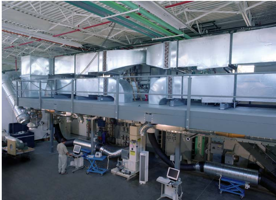
Figure 4. Wide-angle view of NREL's Advanced HVAC Systems Laboratory in Golden, Colorado Photo by Warren Gretz, NREL
