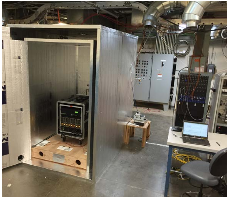
Figure ES-3. Eight servers instrumented at NREL’s Advanced HVAC Systems Laboratory in Golden, Colorado
