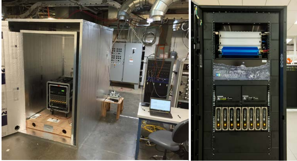
Figure 3. Eight servers instrumented at NREL's Advanced HVAC Systems Laboratory in Golden, Colorado (left) and eight servers installed at NREL's ESIF data center in Golden, Colorado (right) Photos by Eric Kozubal and Dennis Schroeder, NREL
