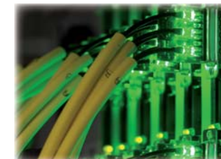
Optical fiber temperature measurement system
