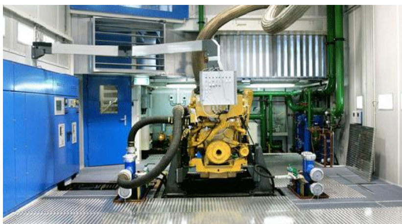
Figure 1: Test bed at Pon Power (courtesy Pon Power)
