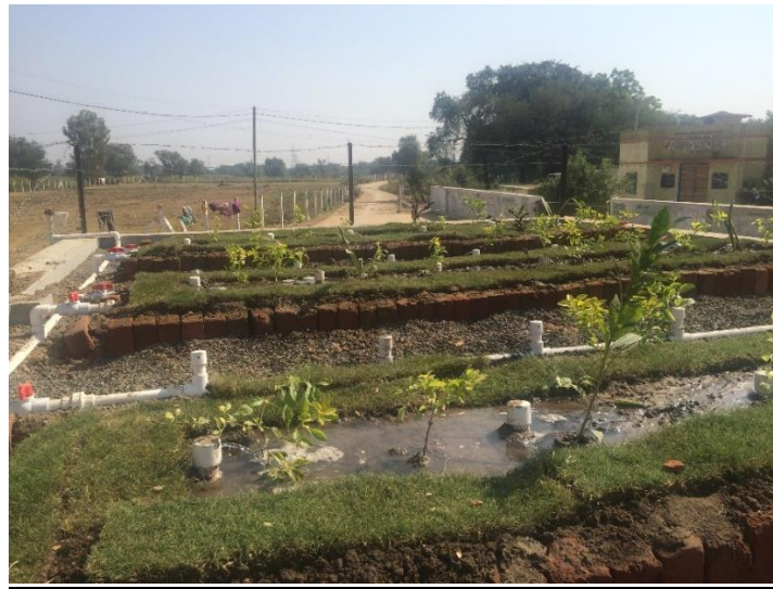
Modified CAMUS SBT Sewage Treatment Facility
